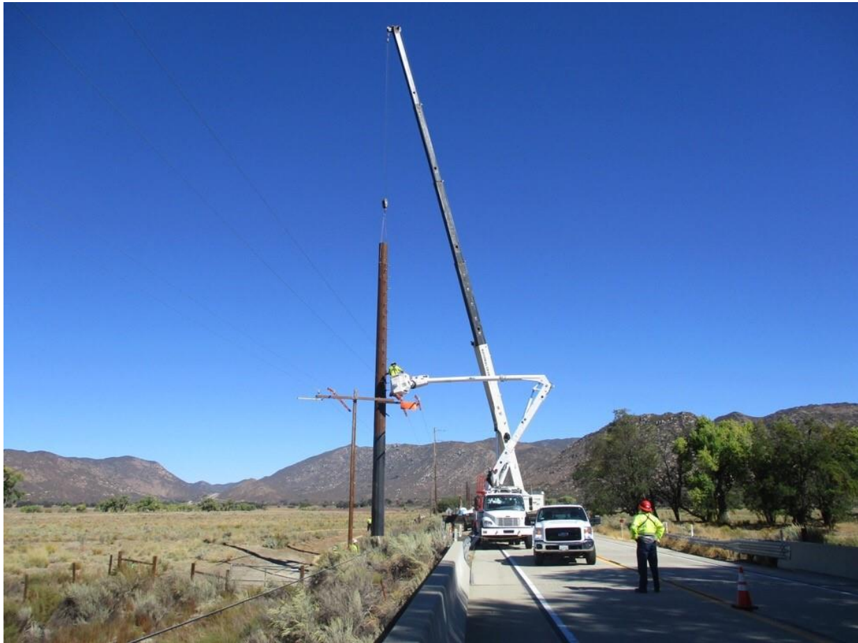
Photo 5: A construction crew spreading wire and installing a new pole at Pole Z40556 (TL 629C). A dedicated fire patrol was present for the work with energized lines in accordance with the CFPPP for the day's stated fire conditions. Traffic control personnel were observed implementing a lane closure along Old Highway 80, and utilizing a pilot car to guide motorists around the construction activity in accordance with APM TRANS-02.
