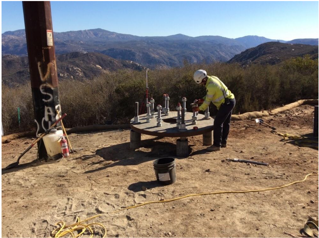
Photo 1: A construction worker observed installing a micropile foundation cap at Pole Z571460 (TL 6957). A complete set of fire tools, including a 5 gallon backpack pump, round point shovel, Pulaski, and 2A10BC fire extinguisher, were located on-site in accordance with the CFPPP (MM FF-1) and APM HAZ-04.
