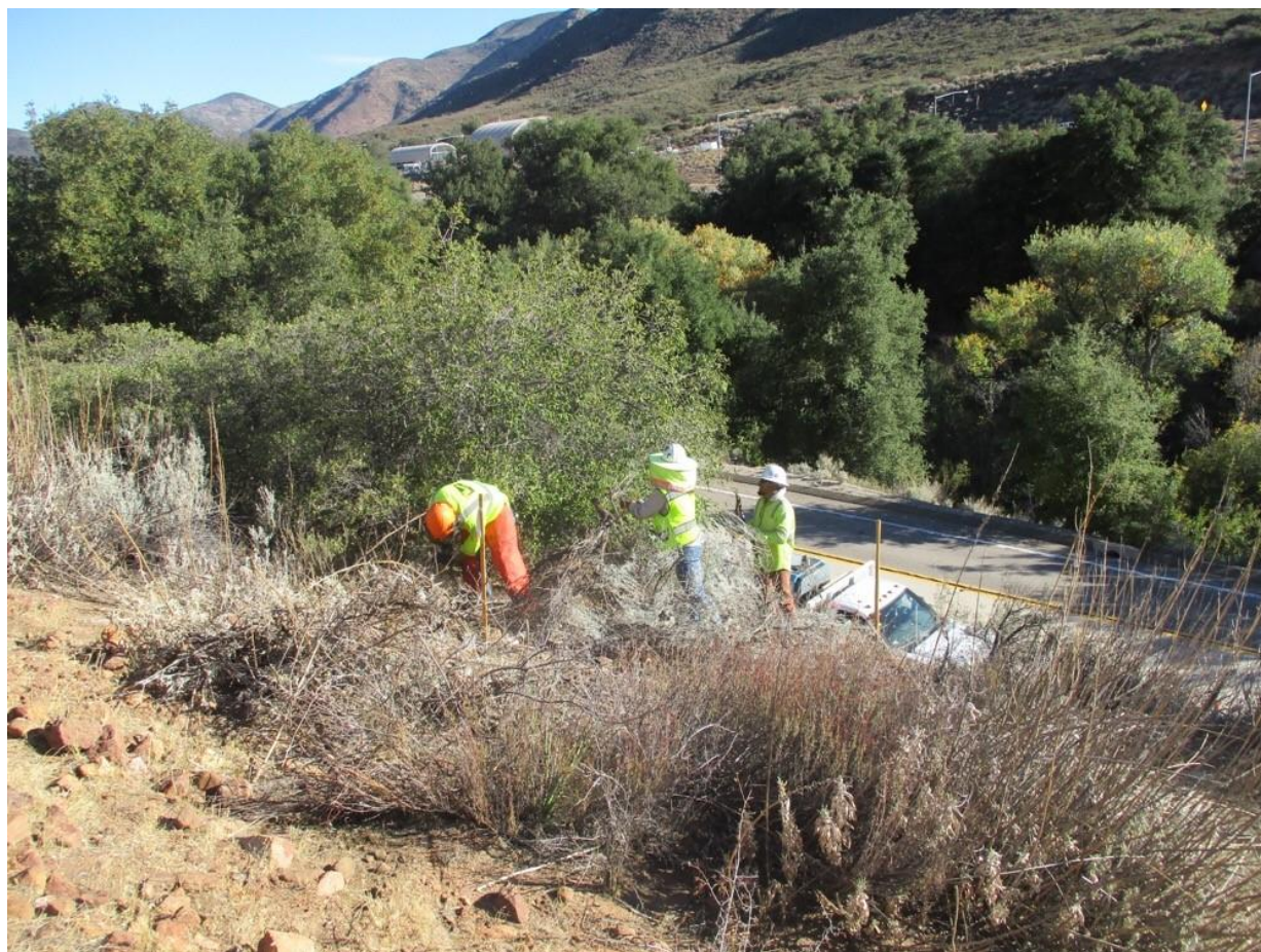
Photo 4: A construction crew observed clearing vegetation within the approved workspace for Pole Z40423 (TL 629C). A biological monitor was present on site for the vegetation clearing work in accordance with MM BIO-3, and was observed communicating with the construction crew about the delineated workspace limits to ensure all impacts to vegetation occurred within the approved workspace in accordance with MM BIO-1.
