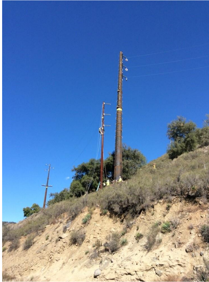
Photo 6: A construction crew observed cutting an existing/old steel pole for removal at Pole Z118088 (TL 682). A dedicated fire patrol was present on-site for the hot work as required by the CFPPP (MM FF-1) for the day's stated fire conditions.
