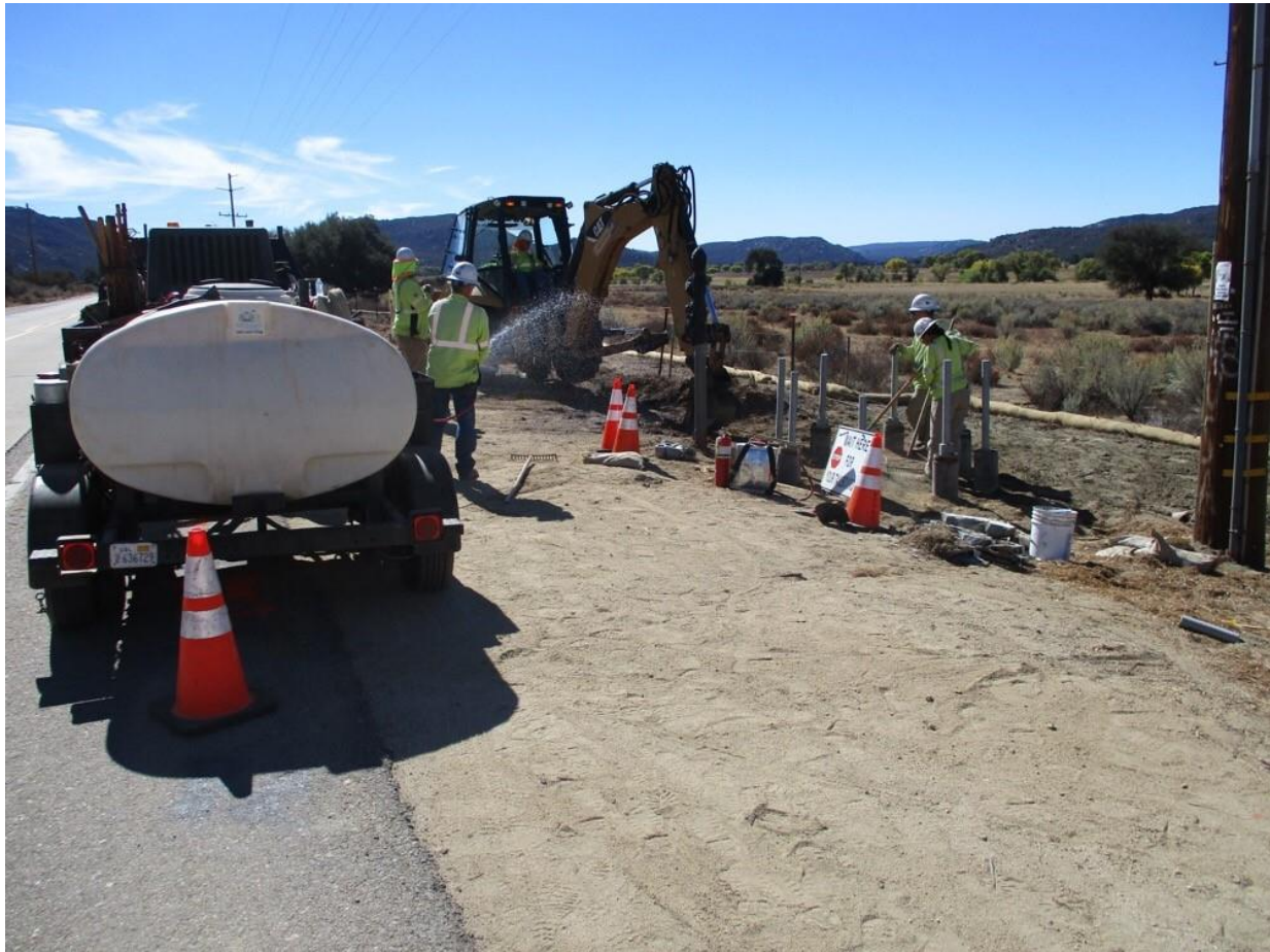
Photo 2: A construction crew observed trenching for the installation of grounding at Pole Z40535 (TL 629C). As required by the CFPPP (MM FF-1) for trenching work during fire conditions for the day, the construction crew was equipped with 150 gallons of water (with pump and hose), and was observed watering the area to prevent ignition. The area was also watered to reduce dust emissions in accordance with APM AIR-02 and APM AIR-05.
