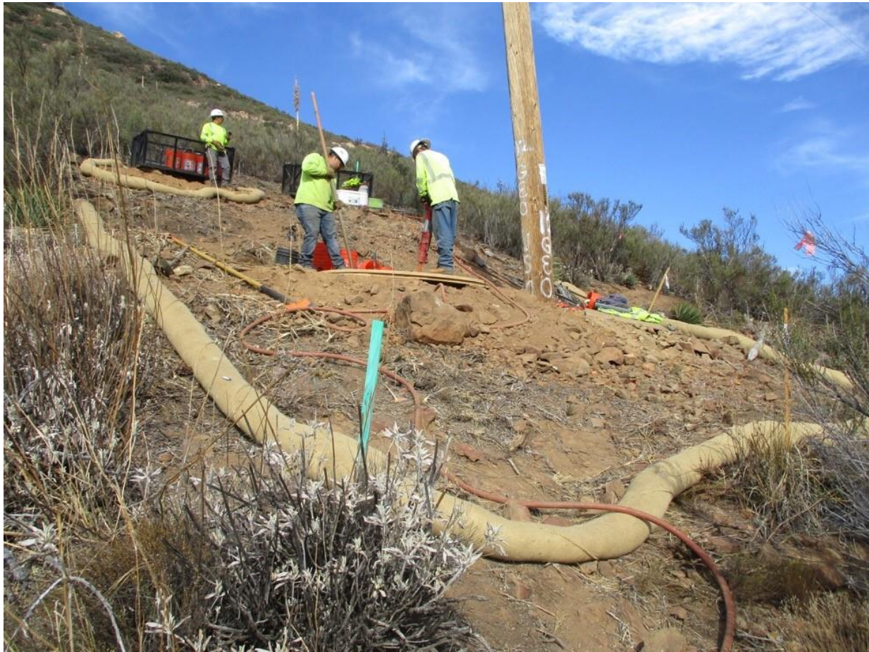
Photo 3: A construction crew observed excavating a direct-bury pole hole at Pole Z40464 (TL 629C). Sediment control BMPs (fiber rolls) were observed along the downslope side of the workspace to prevent off-site erosion in accordance with the ECP and SWPPP (MM HYD-1, APM HYD-09, MM BIO-7).
